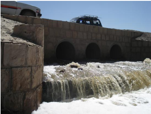
Figure 6-131 Flow downstream from the road culvert at Bani Garmouz
