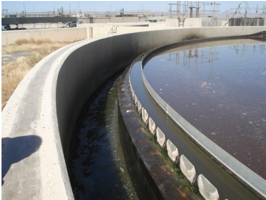
Figure 6-117 Treated wastewater flowing out from the trickling filter
