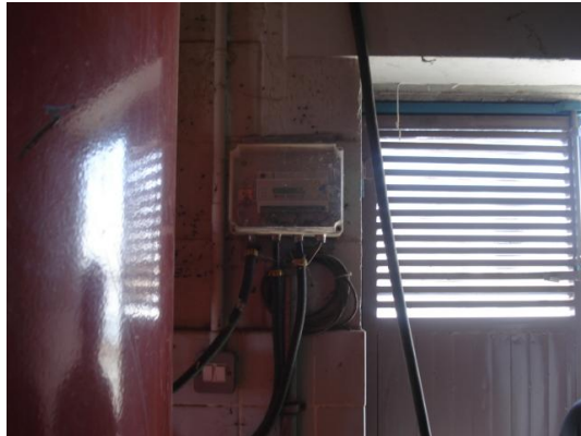
Figure 6-124 Data logger for the ultrasound device on Sana'a WWTP
