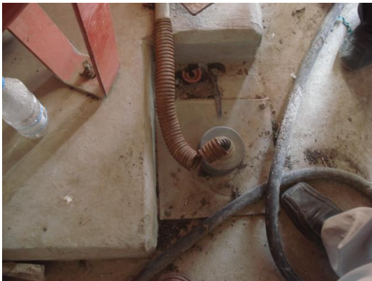
Figure 6-123 Ultrasound surface water measuring device in Sana'a WWTP
