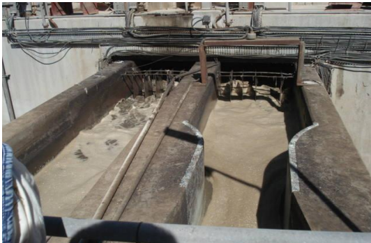
Figure 6-113 Inlet channel for raw sewage and the parshall flume
