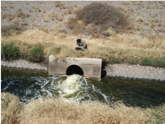
Figure 6-121 Outlet of Sana'a WWTP
