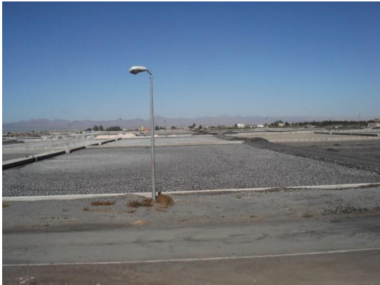
Figure 6-118 Sludge drying beds in Sana'a WWTP
