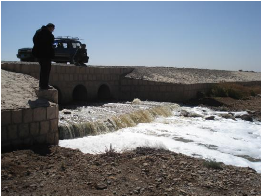
Figure 6-130 Flow downstream from the road culvert at Bani Garmouz
