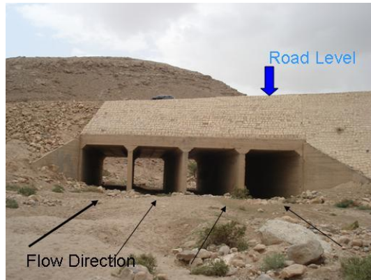
Figure 6-60 Front view of the box culvert structure at the intersection of the Wadi Khulaga main floodway and a highway. Coordinates of the crossing structure are: for the left side: UTME=437089 and UTMN=1734937, and for the right side: UTME=437117 and UTMN=1734951, at an elevation of 1925 m (AMSL)
