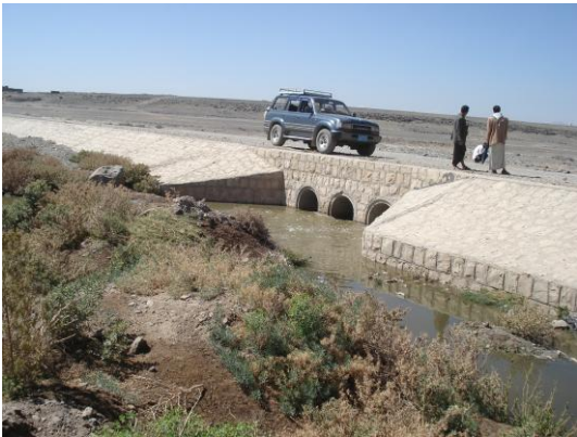
Figure 6-127 The road culvert in the Bani-Garmouz area. Al-Mosayerka Dam is 1.5 km downstream
