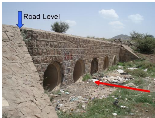
Figure 6-6 Side view of the crossing structure at the location of the main monitoring station in Sanhan
