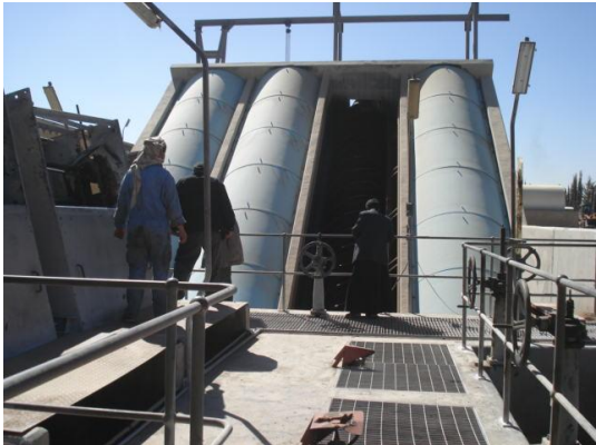
Figure 6-114 Lifting pumps inside Sana'a WWTP
