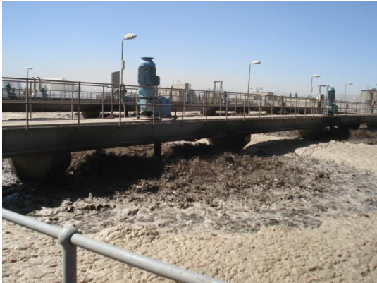
Figure 6-115 Aerators at work inside the aeration basins of Sana'a WWTP
