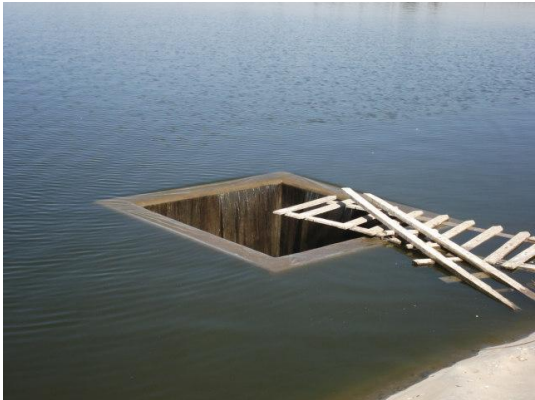
Figure 6-120 Rectangular siphon of the Sana'a WWTP outlet
