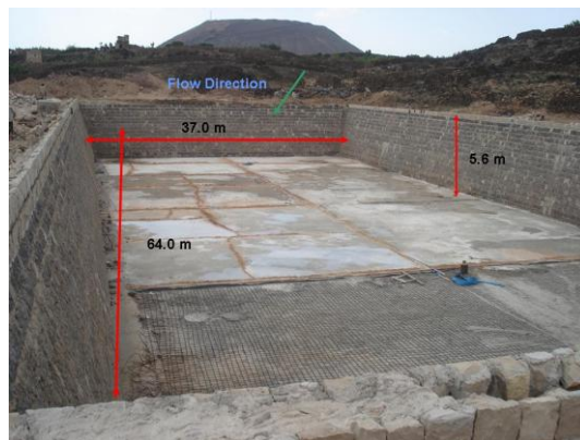
Figure 6-79 Dimensions of the reservoir (under-construction) in the main stream of the Wadi Iqbal floodpath. Coordinates are: 1714085 and UTM E 408986
