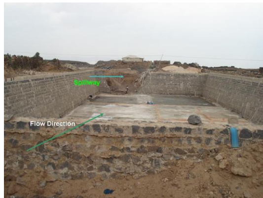
Figure 6-81 General view of the reservoir showing the location of the spillway and the flow entrance structure
