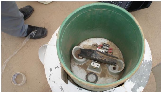
Figure 2-21 Top view for the water leveler, bubble leveler and electrical board
