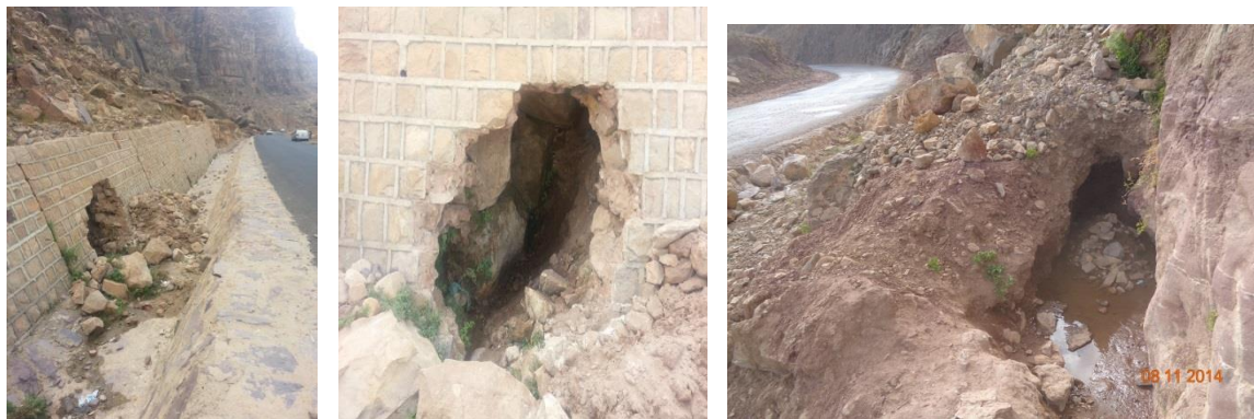
Figure 22. & 23. & 24. Neglecting spring source requirements lead to land users to dig the retaining wall (picture at the middle and left) to follow the spring flow which disappeared after the road construction and hill protection works. In other instances springs are re-excavated (picture on the right) after erosion
