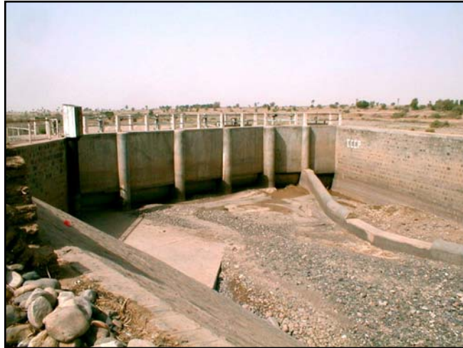
Faleg Weir Head Reg. & Scour Sluice
