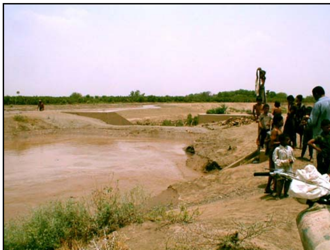
Mawi Canal, Temporary Earthen Check upstream of Drop Structure and Outlets, 8 August 2002
