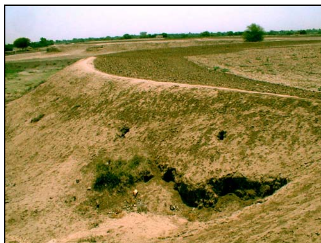
Mawi CA. Holes in field embankment & ploughed inner slope of bund to try and prevent bank failure by sealing holes. 8 th August 2002
