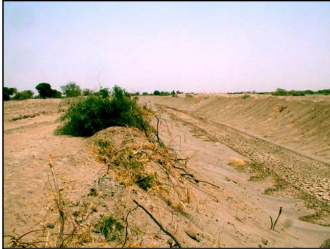
Manasira Primary canal with wind blown sand accumulation, 14 August 2002
