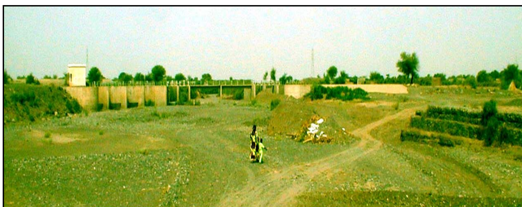
Weir 4 Left (Wadi Ain) Side with offtakes to Bira (L) & Gerab (R) Canals. Weir 4 Right (Wadi Nasery) side is located to the right of the earthen bund out of the picture. 8 th August 2002
