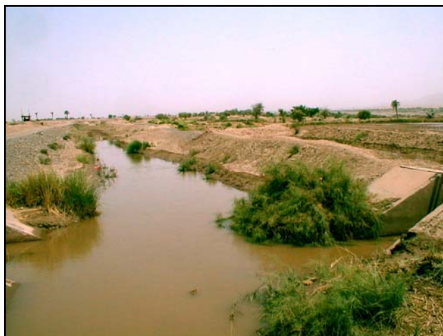
Water joining the Al-Arais Main Canal just upstream of the P19 and P22 turnouts, 12 August 2002
