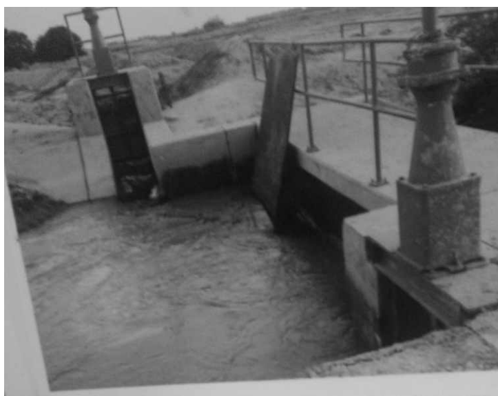
Figure 8.4: The wooden plank used to divert water to the gate that takes some floodwater to person 82
