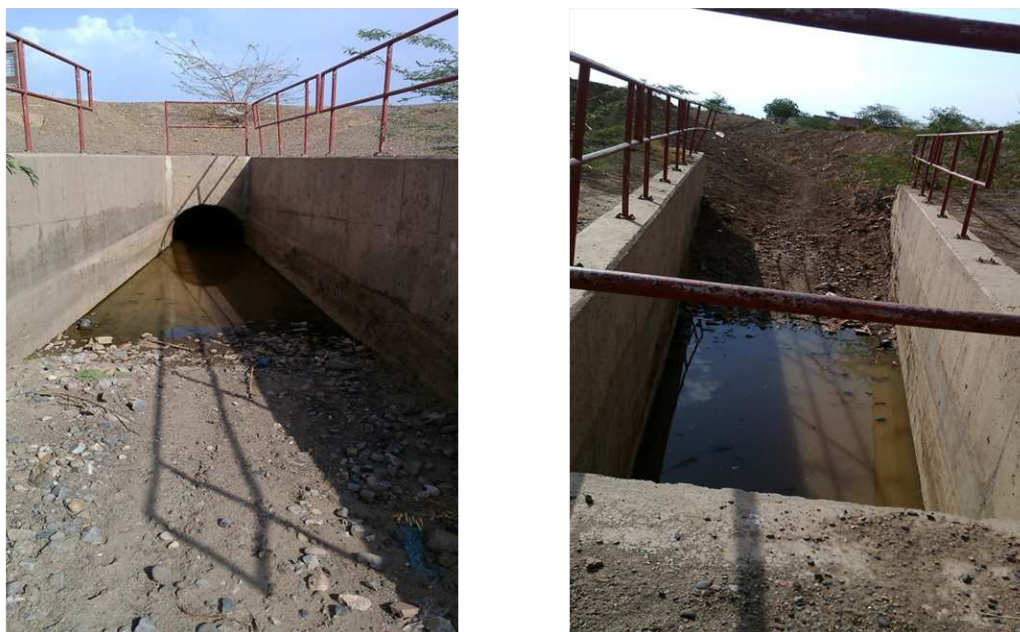
Figure 8.5: Culvert design leading to sedimentation
