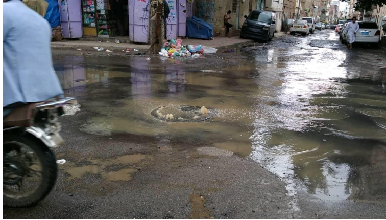
Figure (4.5): The overflow of the sewage system in the Ma'ain District in Sana'a city
