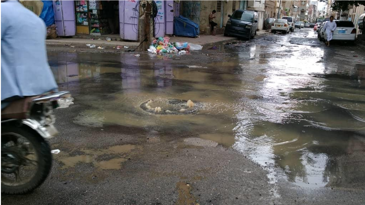
Figure (A6-9): The overflow of the sewage system in the Hayel region in Sana'a city
