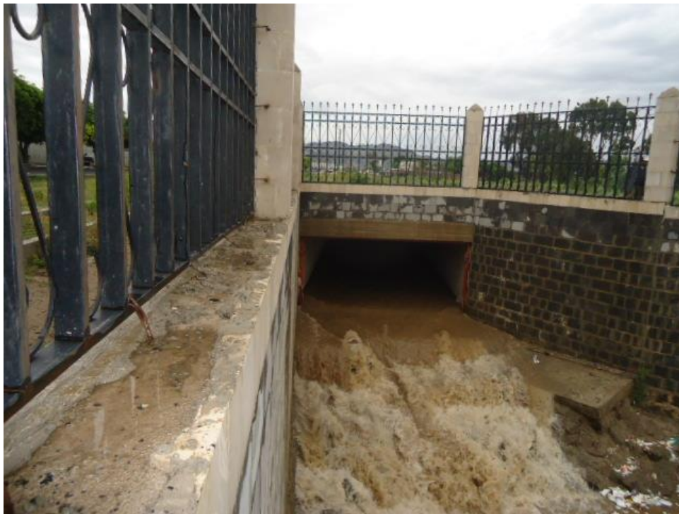
Figure (4.19): Concrete channels to drain rainwater pour into the stormwater retention pond in Al- Sabeen district
