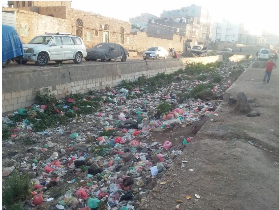
Figure (A6.13): Wastes and sediments in rainwater channel in Ma'ain district.
