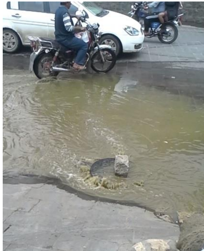
Figure (4.6): The overflow of the sewage system in the Al-Saylah channel close to the old Sana'a city
