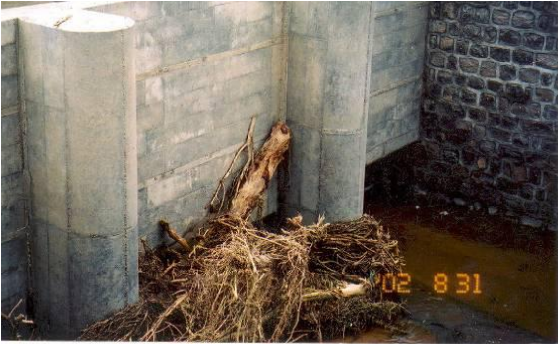
Figure 2-4 : Intake partly blocked by trash
