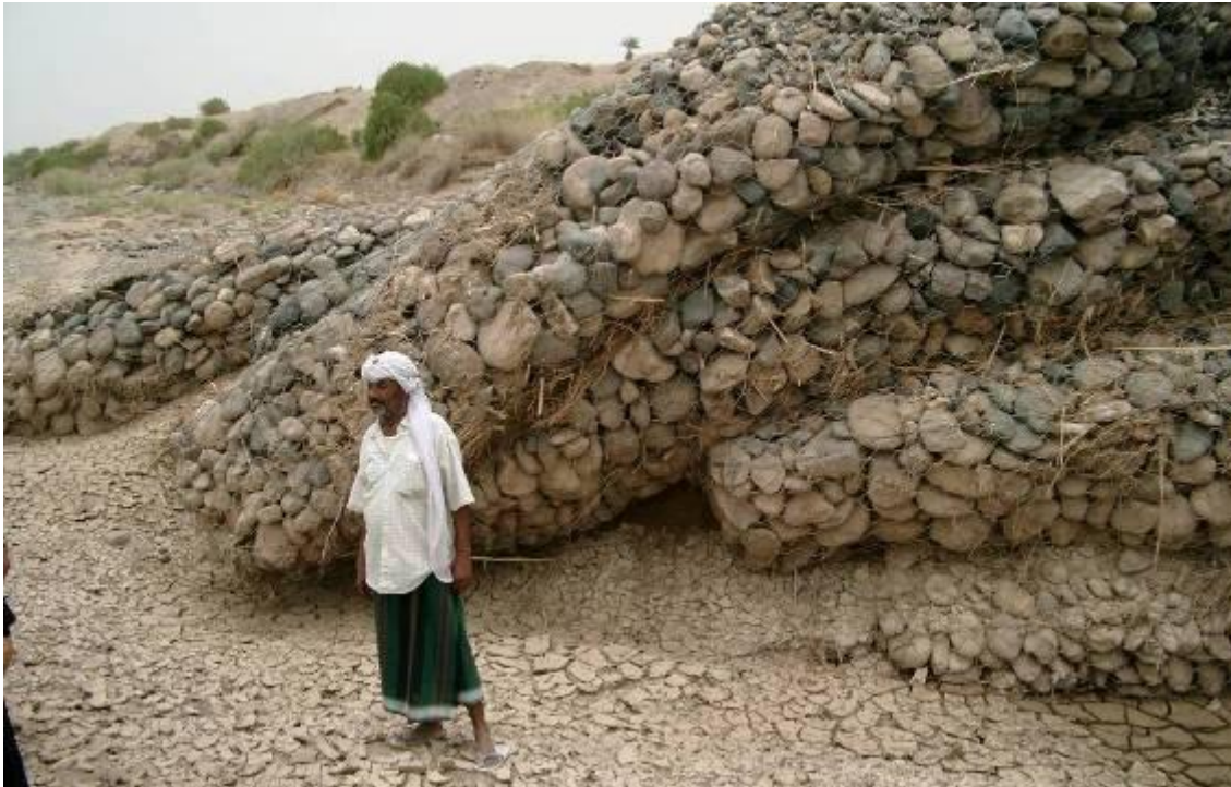
Figure 3-1 : Collapsed nose of spur
