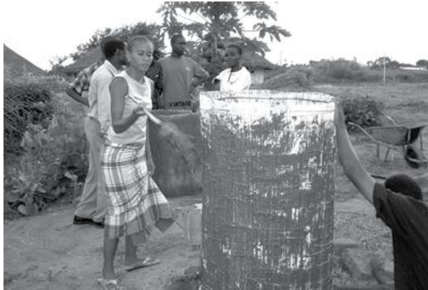
Figure B-2. Painting both the inside and the outside of the cylinder straw mat tank using water and cement solution and large brush
