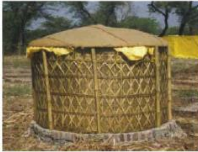
Figure B-3. Bamboo tank developed by ARTI in Pune, India, uses a polythene sheet in a basket structure
