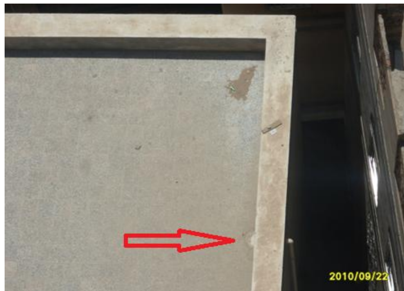
Figure 4 - 5. The place of sampling (cleaning gutter), Massjed AL-Qader
