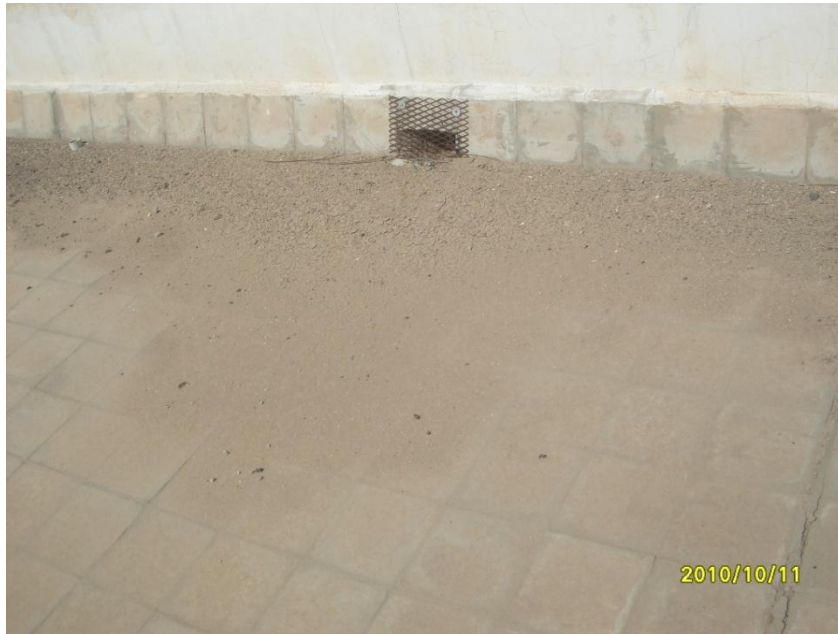
Figure 5 - 11. Accumulated dust in the roof of Aminah bent Wahb School, Existing system.
