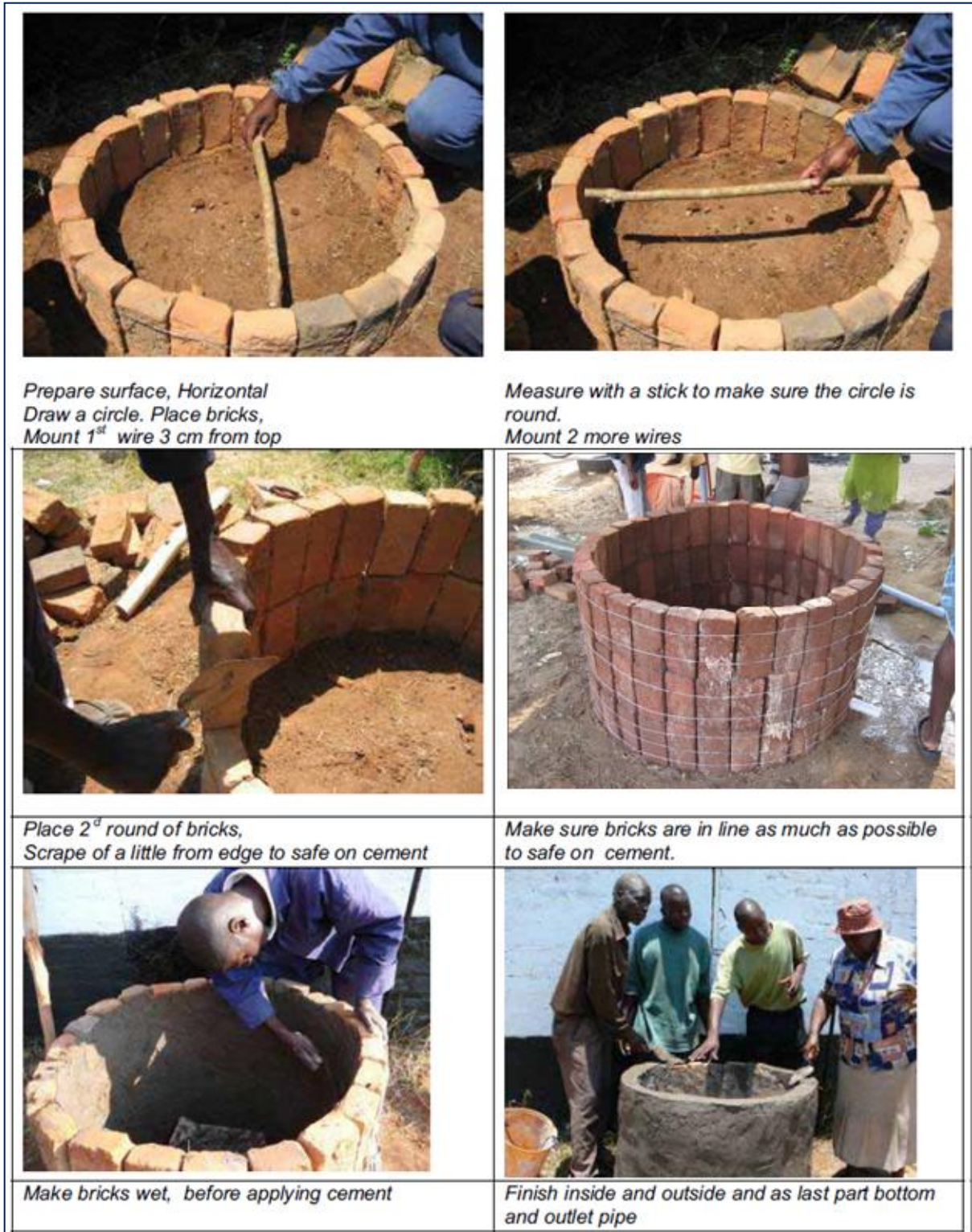
Figure (A-1) Brick cement tank (400 Liter) Construction Used in Arrakis and CI projects
