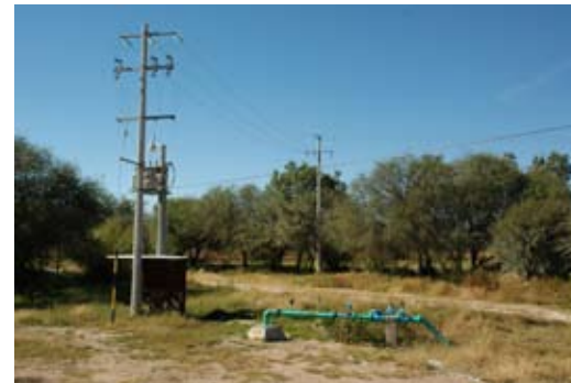
Electricity supply and bore well, Guanajuato, Mexico
