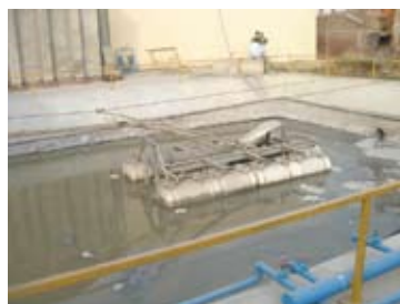
Primary treatment of tannery waste water
