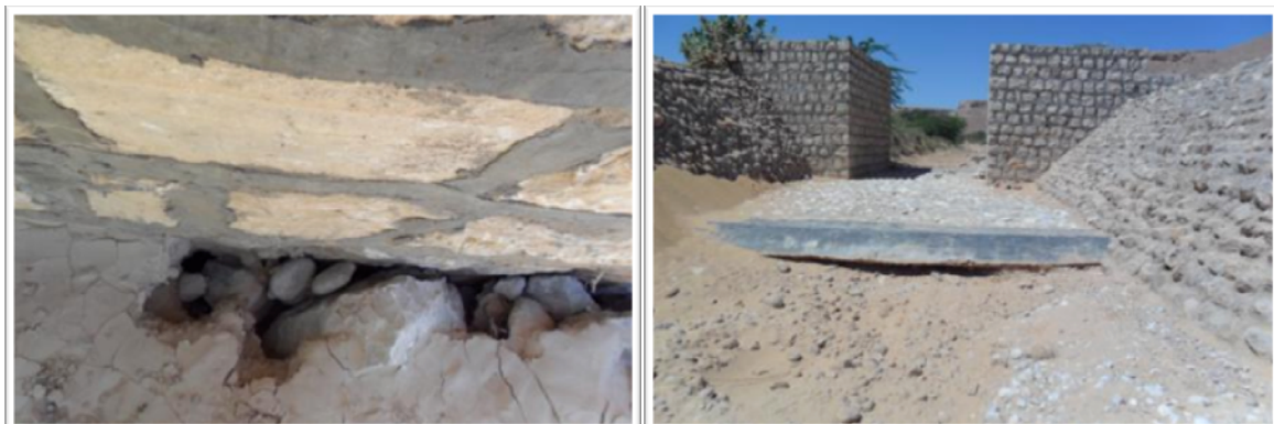
Deferred maintenance in addressing scour or repairing cracks can lead to much larger damage in the spate systems
