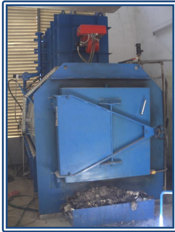
Figure 3-5 Al-Thawarah Hospital Incinerators –Sana’a Capital
