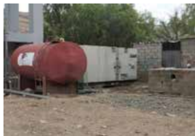
Figure 26 example of on-site diesel tank at a water well
