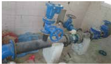
Figure 17 Pumping and pressure management units in Hudaydah network
