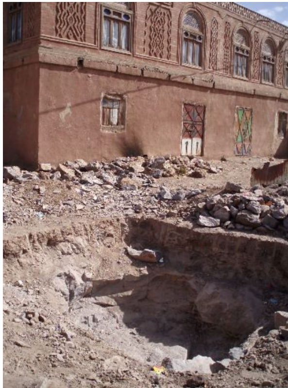
Photo 5 Cess pit (bayaara) being excavated next to the house. It will be unlined, but covered when finished
