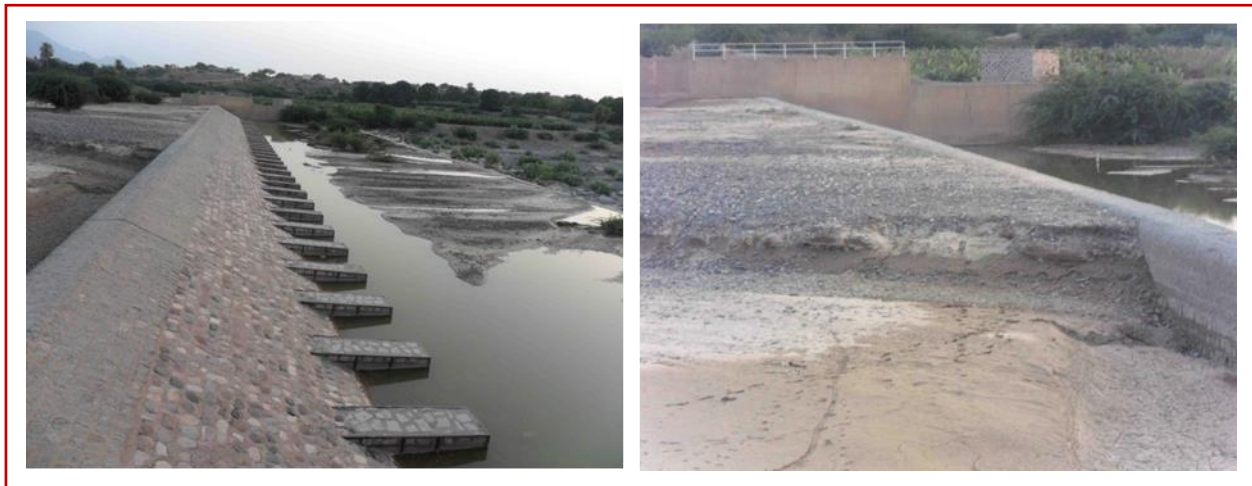
Figure 2.8: Photos shows the raised body of weir 1 and the current sediments accumulation.
