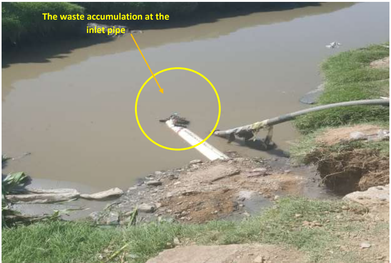
Photo (9): The waste accumulation at the inlet pipe - Source Own Representative
